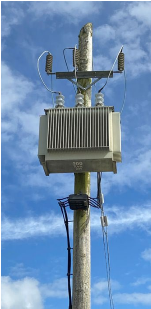
Fig. 7 200kVA Pole Mounted Transformer
