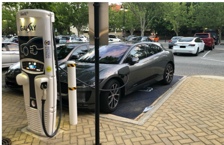
The complexities introduced by EV charging infrastructure and EVs requires further testing, especially as EVs are expected to drive major load growth in distribution networks.
