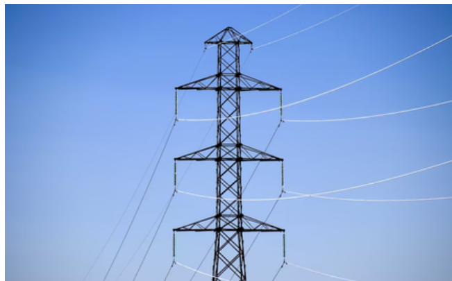
Planned transmission lines have emerged as the front in resistance against the transition.(ABC News: Peter Curtis)
